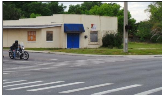
Boarded windows, overgrown weeds, and debris should be avoided in vacant structures.
